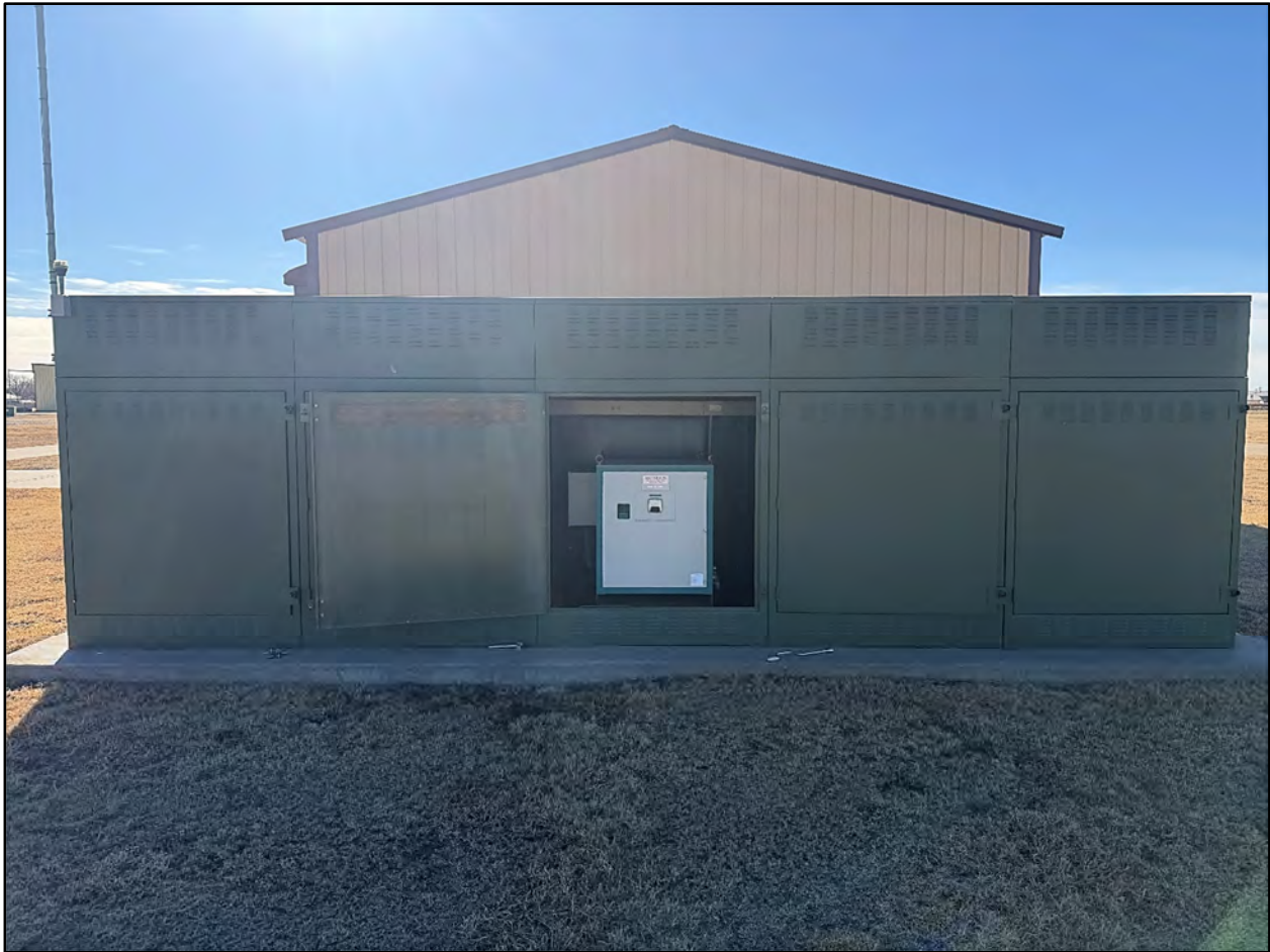
Figure 5: Existing Metal Enclosure containing the CCR for Runway 18-36
