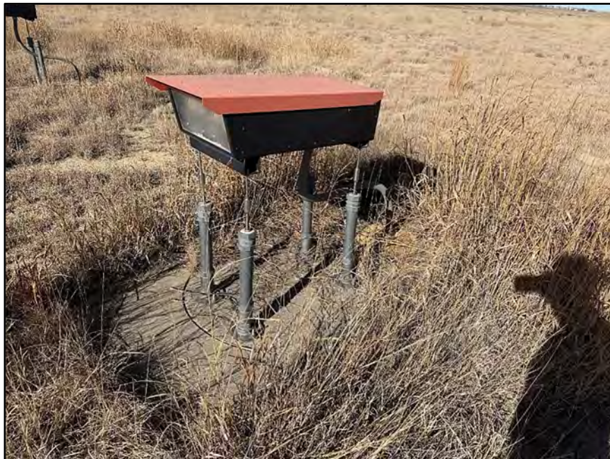
Figure 4: Existing PAPI Unit
