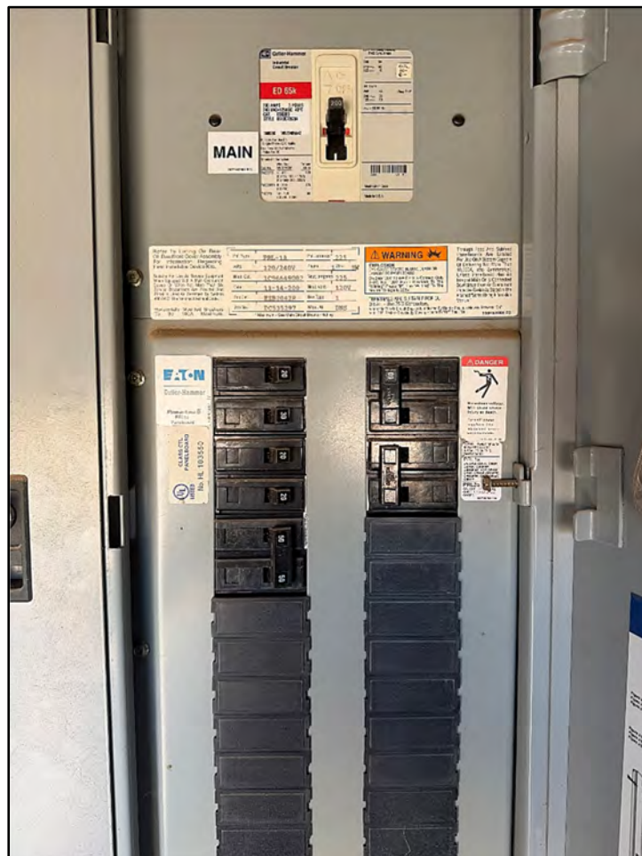
Figure 7: Existing Circuit Breaker Inside the Metal Enclosure
