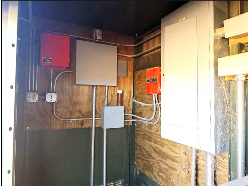
Figure 6: Existing Electrical Controls within the Metal Enclosure
