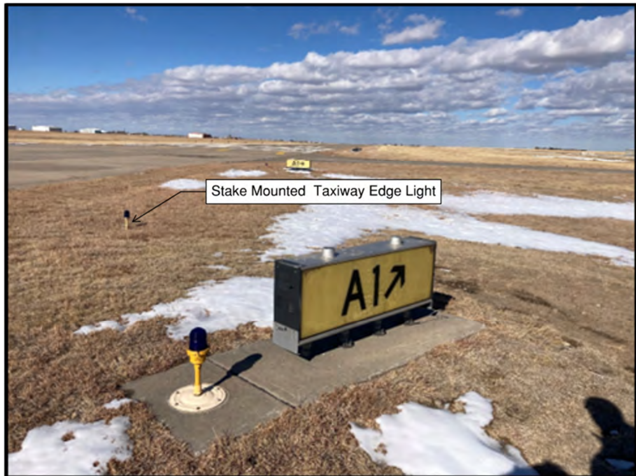
Figure 2: Stake-Mounted Taxiway Edge Light and Taxiway Guidance Sign
