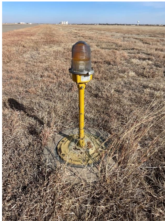
Figure 1: Existing Runway Edge Light
